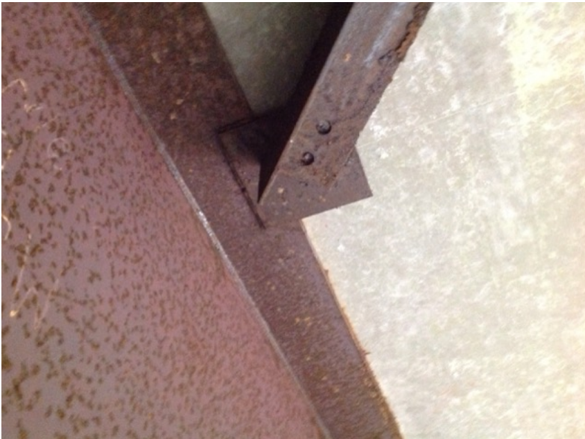
missing bracing bolts
