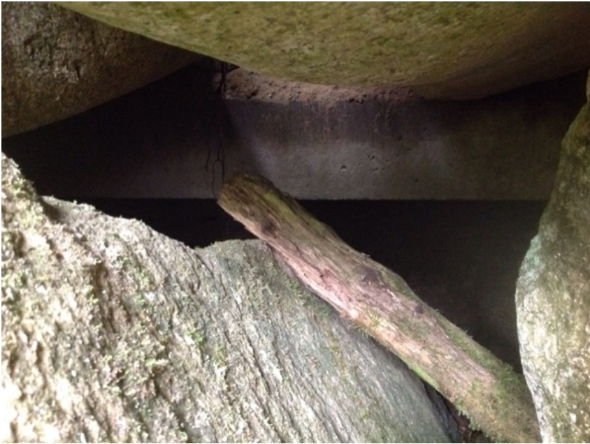
right bank downstream precast footing undermined -approx 400mm
