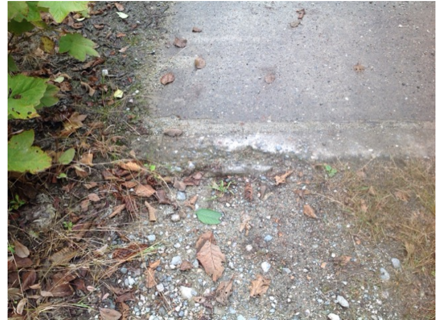
damage to left bank ballast wall
